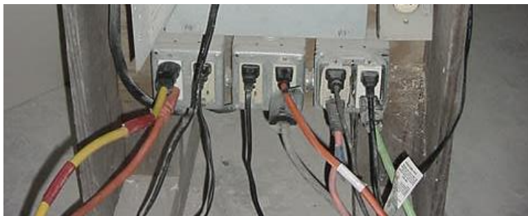
Common temporary set-up of electrical panel with GFCI outlets found on a construction site.
