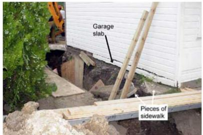
Two views of the scene of a fatal trench cave-in. Notice there is no protection in place to avoid cave-in hazards.
