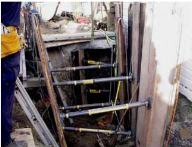
Scene of a fatal trench cave-in after cave-in protection was installed to safely remove the deceased worker.
